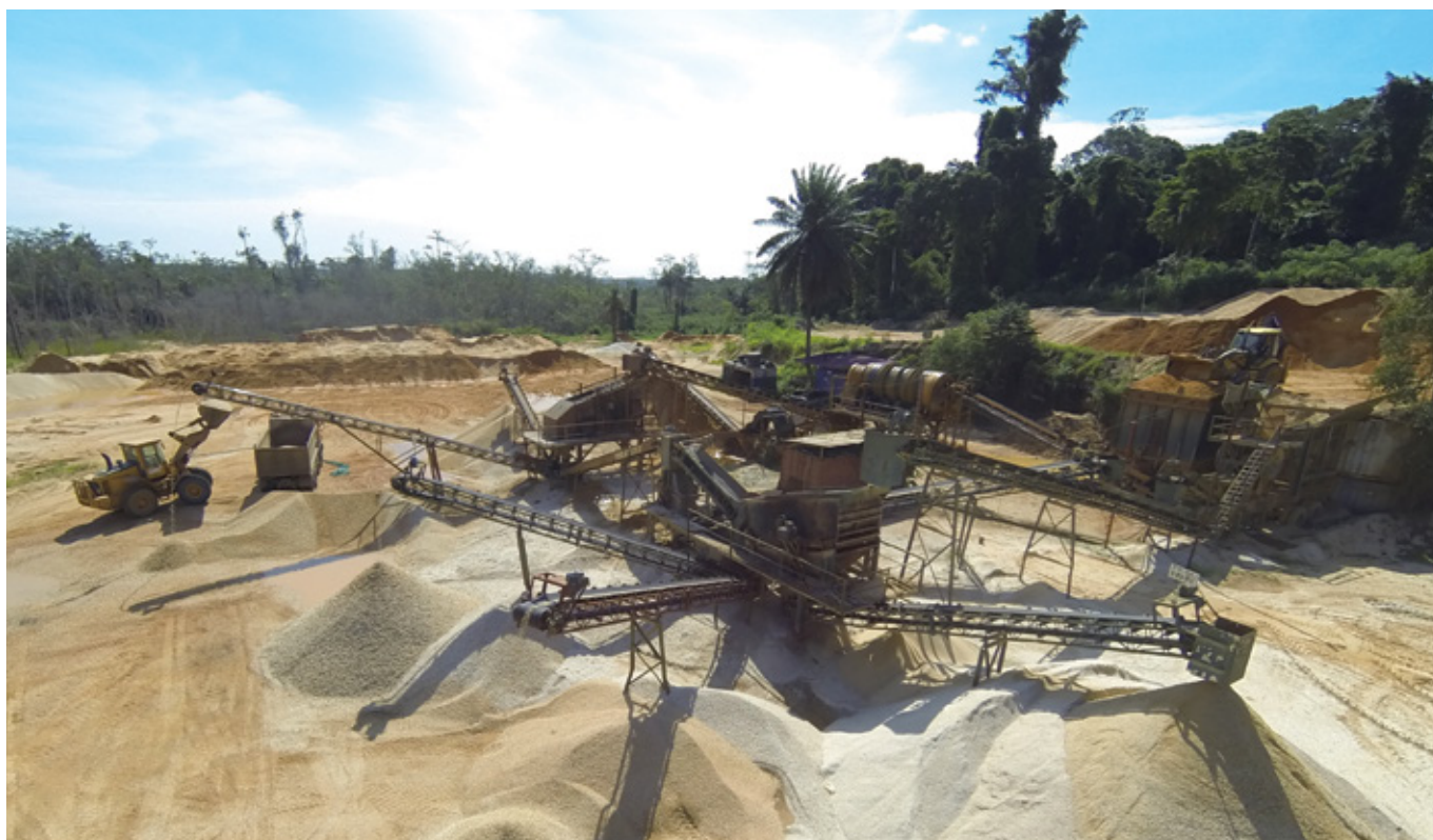
Centro Industrial de Cotchiloango – Central de Britagem, Cabinda. Centre Industriel de Cotchiloango – Central de Broyage, à Cabinda. Cotchiloango Industrial Center – Crushing Plant, Cabinda.
