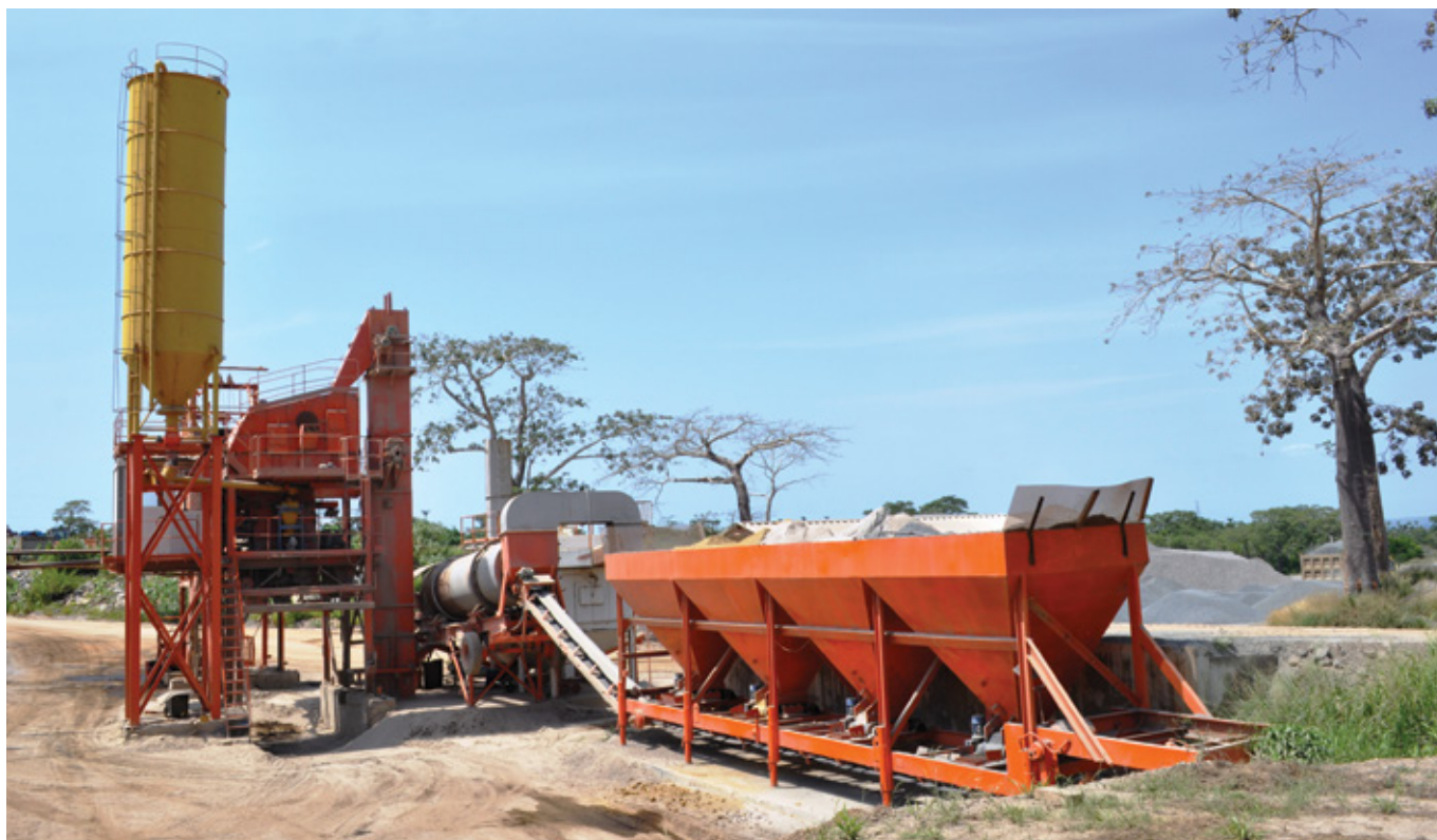
Centro Industrial do Caxito – Central de Misturas Betuminosas, Bengo Centre Industriel de Caxito – Centrale à Enrobés Bitumineux, à Bengo. Caxito Industrial Center – Asphalt mixing plant, Bengo.
